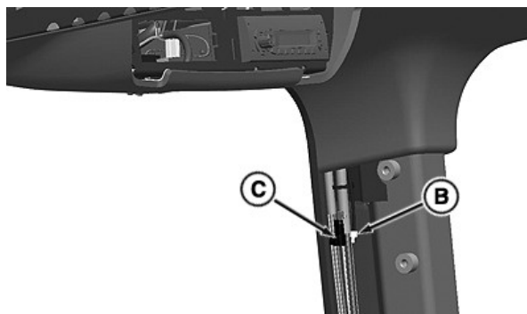
Antenna Coaxial Cable And Business Band Radio Power/Ground plug Coiled Behind Right Rear Corner Post Cover
